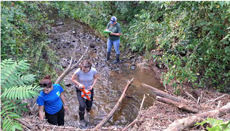
Kristin, Chelsea, and Hannah assessing damaged culverts after a storm in August
